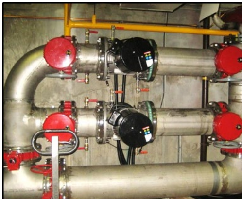
Figure 3.4: Existing UV Disinfection
